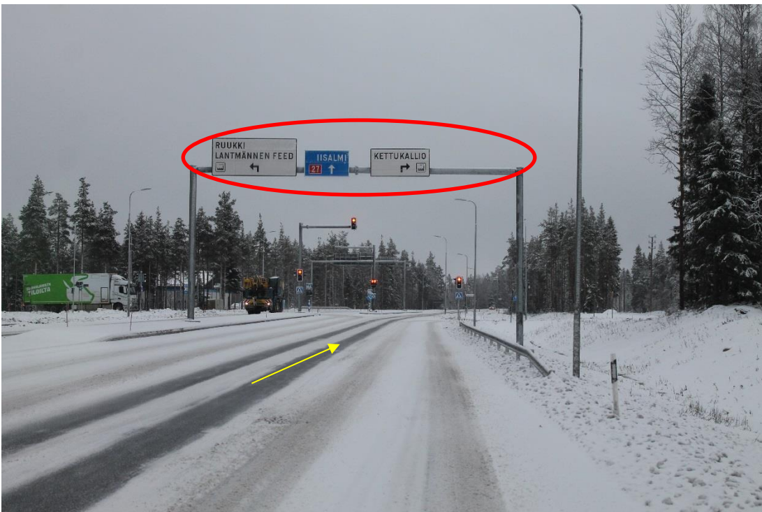
Pic 24/pos 13. Road 27 in Ylivieska. Marked sign need to be removed. Yellow arrow points driving direction.
