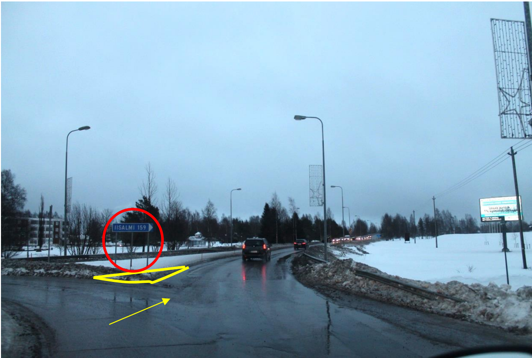
Pic 19/pos 8. Second roundabout in Ylivieska. Marked sign need to be removed. Marked area need to be filled. Yellow arrow points driving direction.
